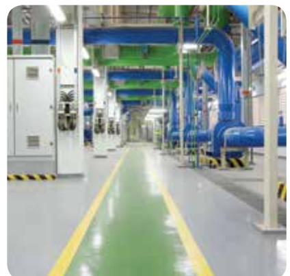
Plant and Maintenance Rooms
